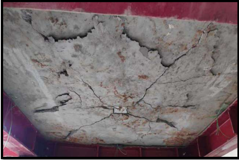
Figure 12: Failure mode of the specimen D150_S200
