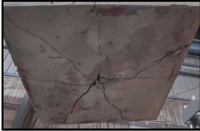
Figure 8: Failure mode of the specimen D170_S200
