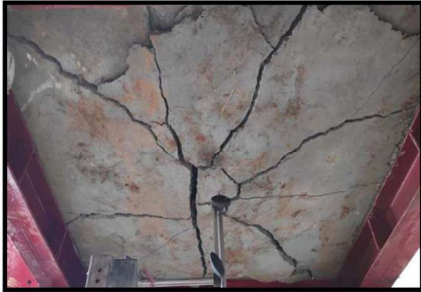
Figure 6: Failure mode of the specimen D170_S150
